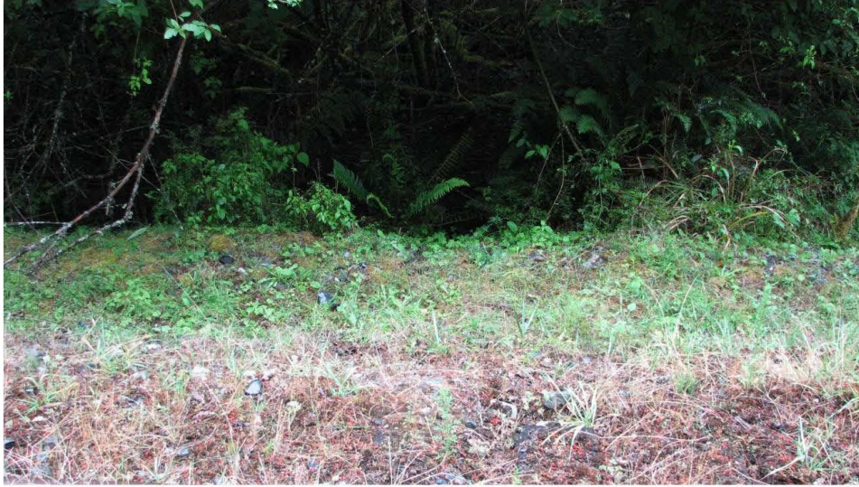
Standing water on parent parcel at bottom of railway right of way
