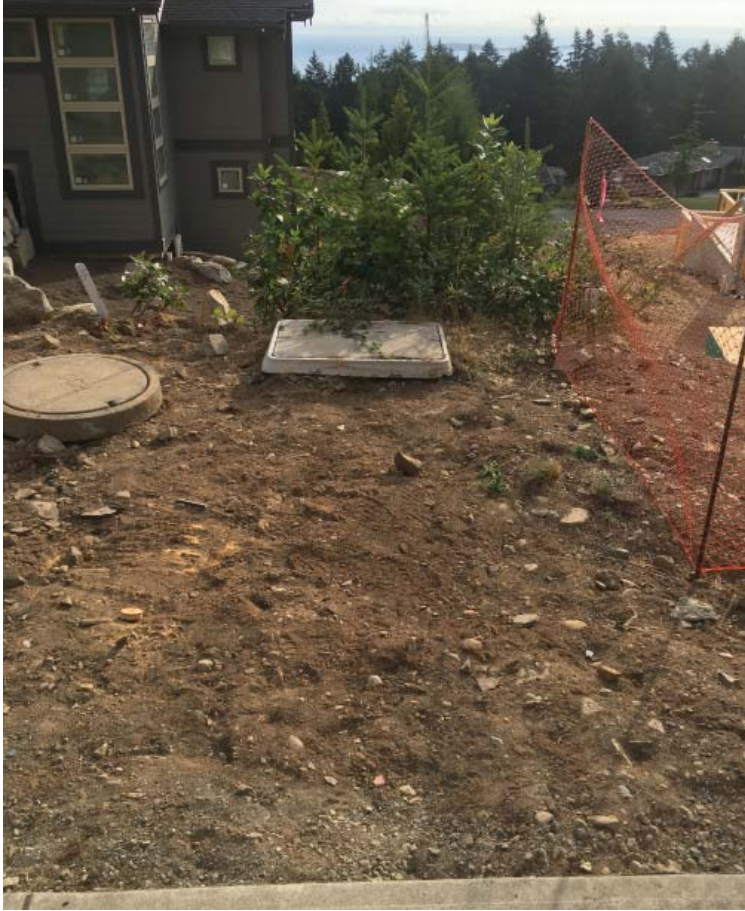
Image 1 (left): Hydro, Tel, Cable infrastructure at top (Bonnington Dr.) end of park land corridor.
