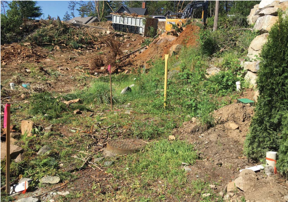
Image 3 (above): Facing west (towards Bonnington Dr.) RDN sewer infrastructure visible. Bedrock and grade change visible behind yellow pipe. Stair work in this area would require monitoring next to existing boulder retaining wall.
