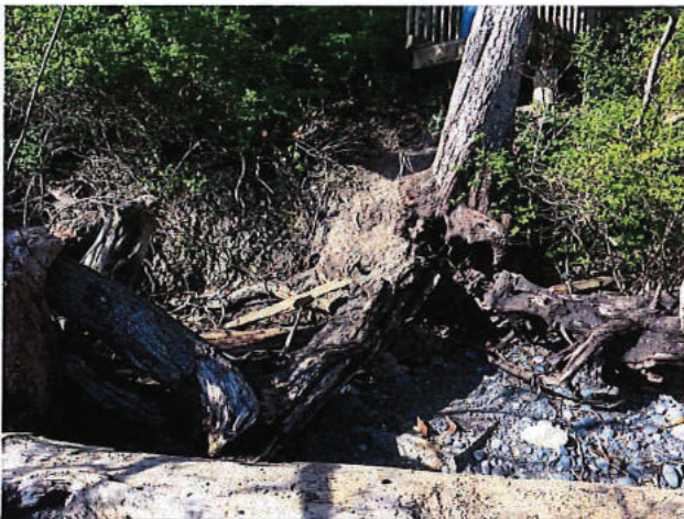
Photo 5 – eroded slope toe and tilted trees below remaining portion of beach access stairs
