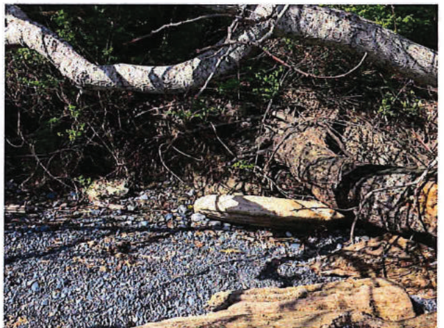
Photo 6 – eroded slope toe and tilted trees below remaining portion of beach access stairs
