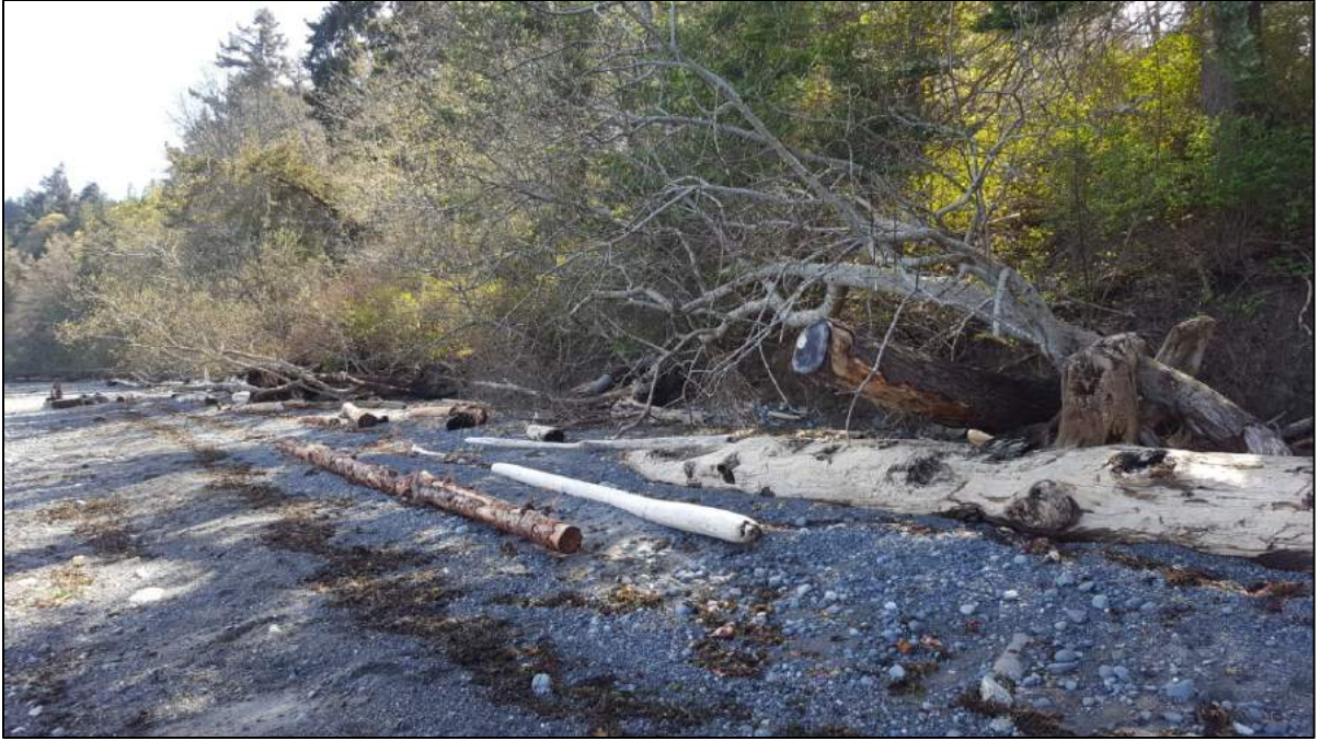
Photo 3. Looking south along the shoreline which is showing the same cut bank at the base of the slope all along the shoreline.
