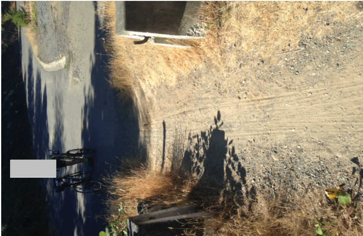
This photo is intended to highlight the hazard of the curbing connector hook; suggest it be cut off or otherwise bent or covered.
