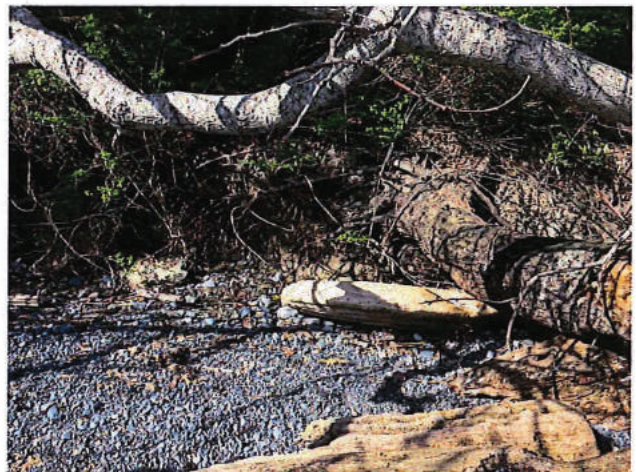
Photo 6 – eroded slope toe and tilted trees below remaining portion of beach access stairs
